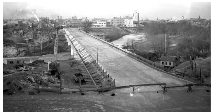
Center Avenue Bridge under construction in 1937. The view is to the west from the Moorhead side of the river.
