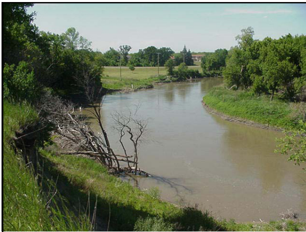
Rotational slump along Red River of the North in Fargo, North Dakota. Note the relationship of this activity to the cutbank and the outside of the river meander (left). (Photo by D.P. Schwert).
